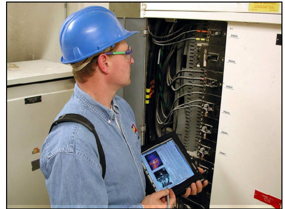
Data capture in the field & information at your fingertips ensures accuracy and accountability as well as eliminating the need for typing up reports after the inspection.
